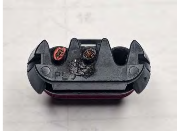
Back of melted plug. Slot on right was where Smaller green wire was removed.
